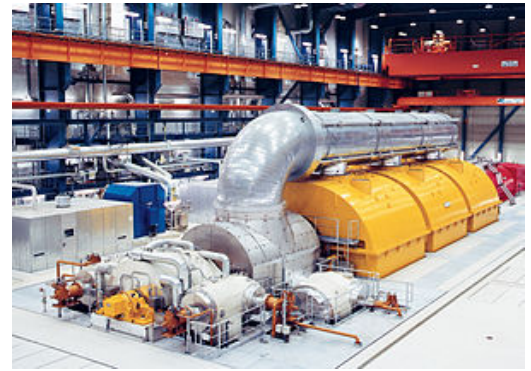
A turbo generator transforms the energy of pressurised steam into electrical energy
